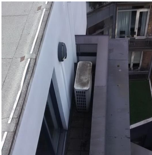
Image 5: Photograph from roof of Zinc House showing existing heat pump at Balcony Level.
